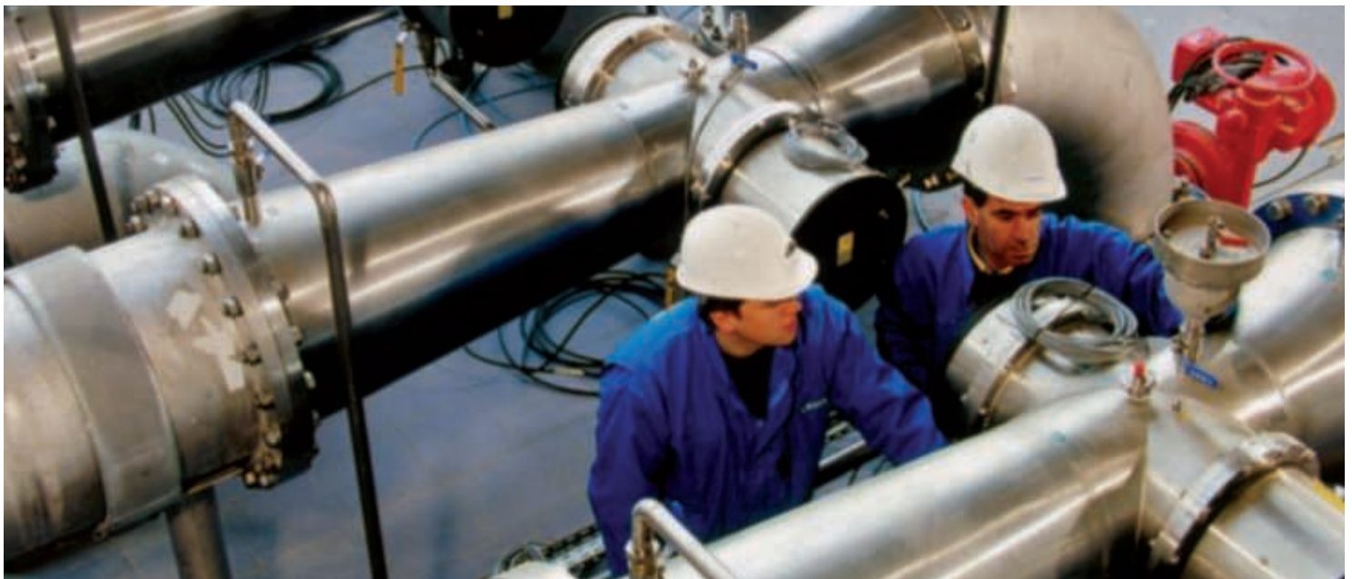
Ultraviolet treatment at the Méry-sur-Oise (near Paris) water plant (SEDIF).
