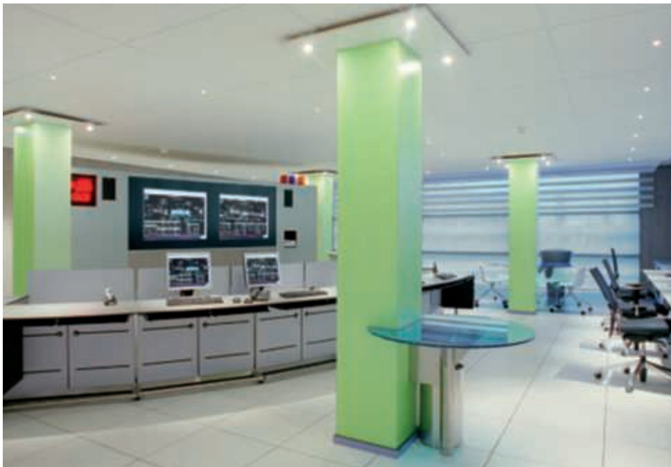
Control station at the Choisy-le-Roi water plant (near Paris).
