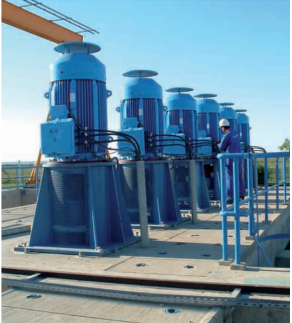
Pumping station near Mechra Belksiri in Morocco.
