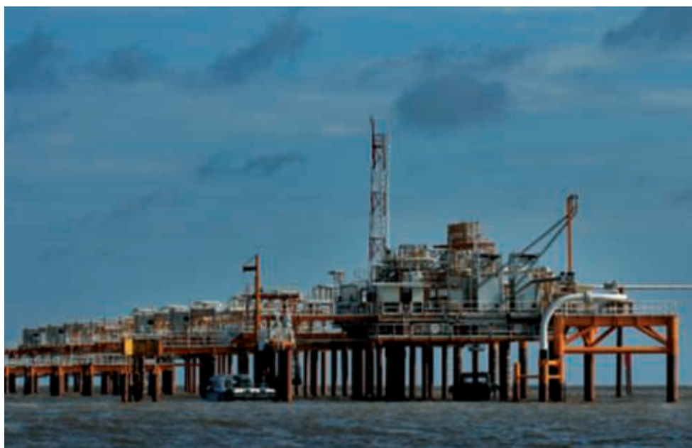
Tunu gas field platform contract awarded to Cegelec by Total.
